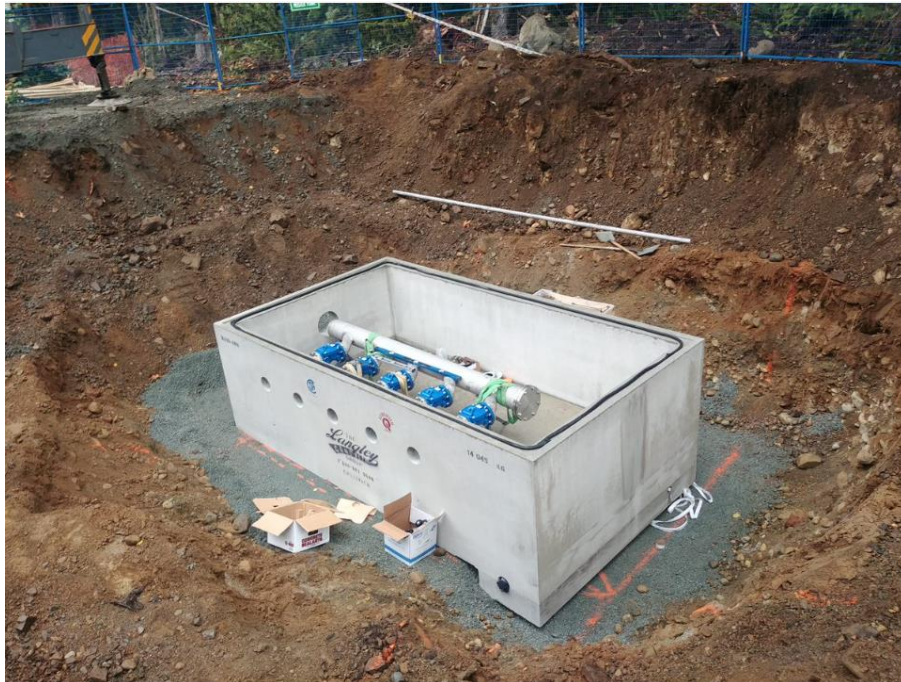
Figure 10 - Influent Manifold Chamber Works (Urban Systems, 2019)
